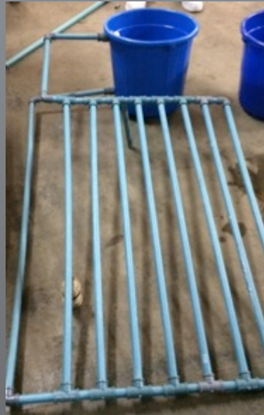
SOLAR WATER HEATING UNIT
